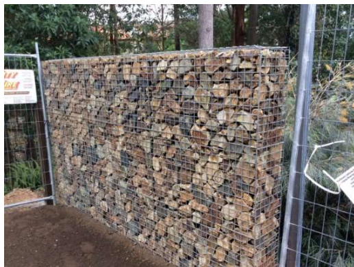
Caged Rock Fence on Galvanised Frame
